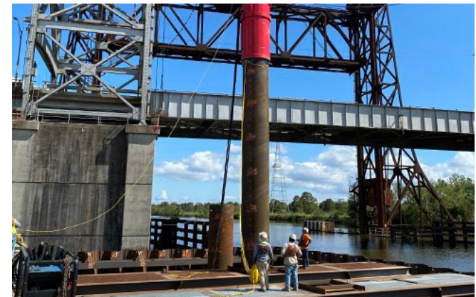
GeoEngineers oversaw the dynamic testing of a 48-inch diameter steel pipe pile for the new bridge's main pier.
